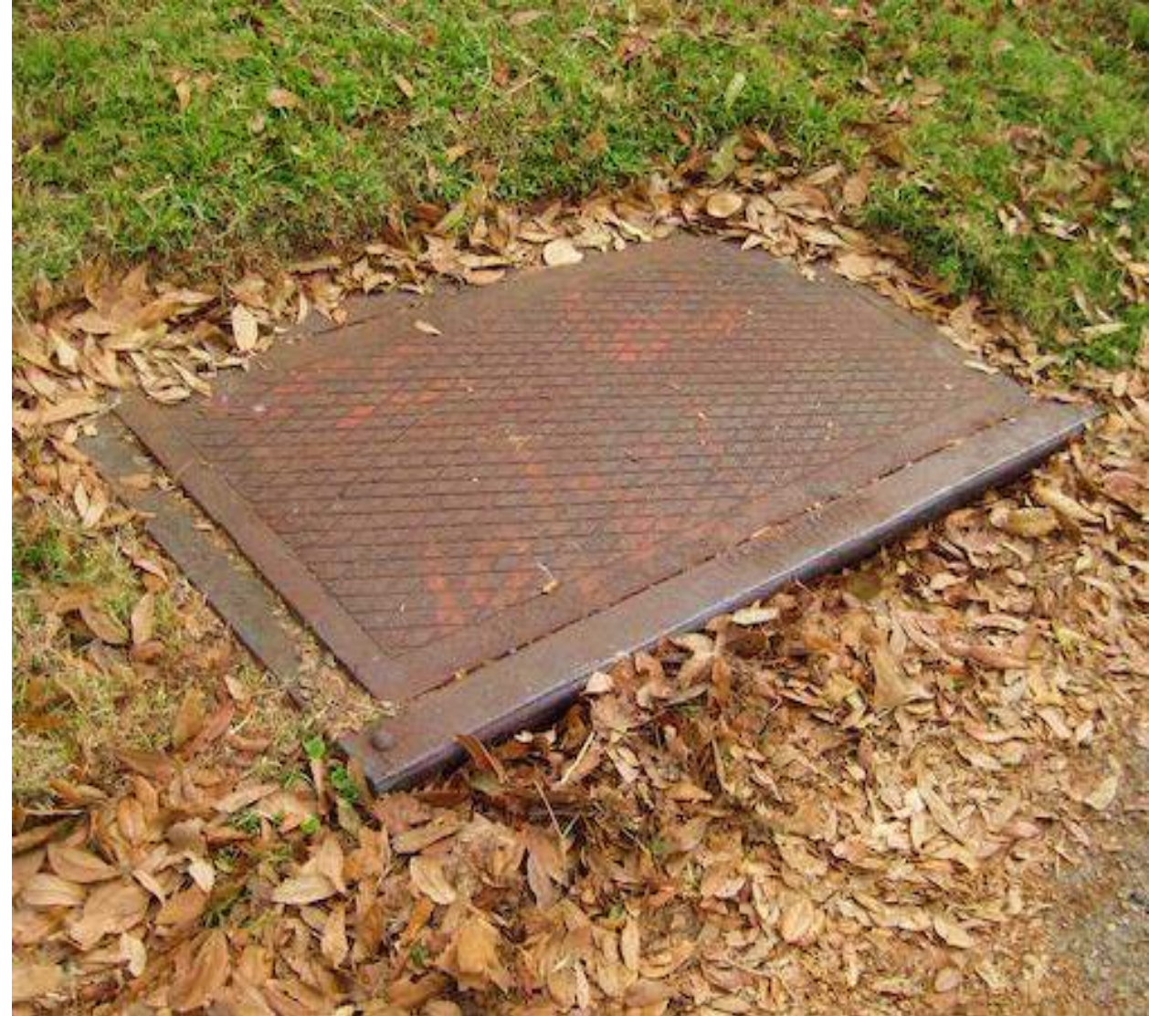
CLOGGED STORMWATER DRAIN SOURCE: STEPHEN C. PICOU
